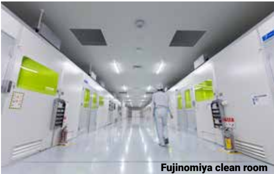
Fujinomiya clean room
